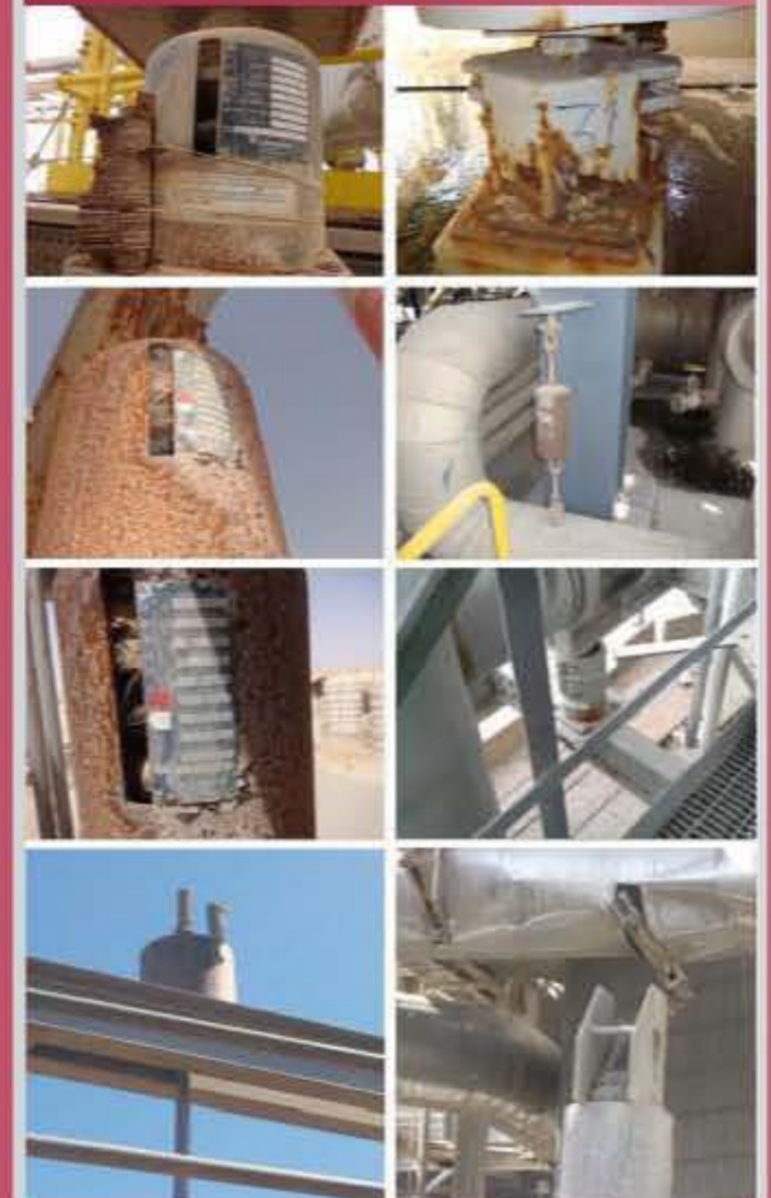
The faults most frequently noted in pipe supports
